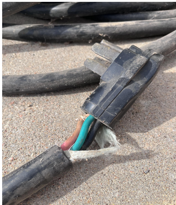
Extension-cable plug end showing the outer jacket/coating pulled away and needing maintenance.
