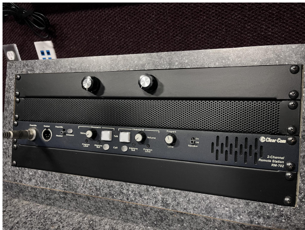
Clear-Com RM-702 2-Channel Remote Station at the front production desk.
