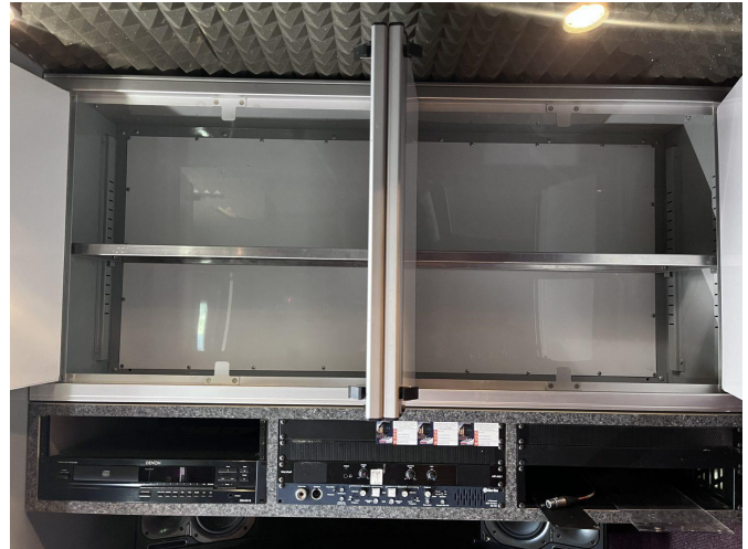
Audio-position overhead cabinets opened; rack equipment and nearfield speakers remain below.
