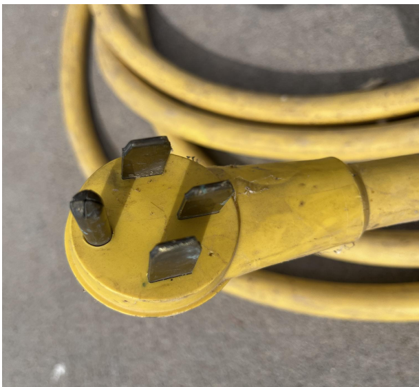
Yellow shore-power cable plug; two approximately 30-ft yellow cables are available.
