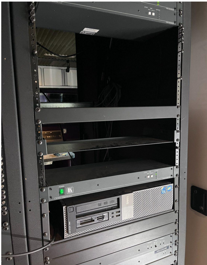
Dell OptiPlex rack-shelf PC, additional Kramer DVI distribution and open rack space.
