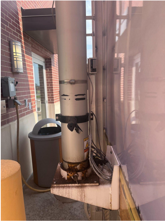
Mast base / mounting area shows significant corrosion and staining.
