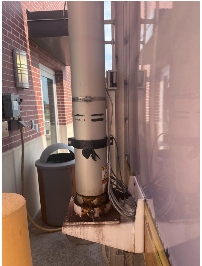
Mast base corrosion and staining.
