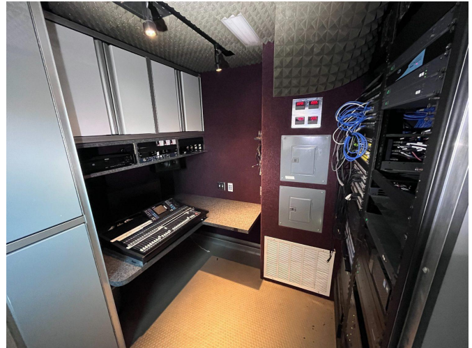
Current audio/engineering area illustrates the remaining fixed racks, electrical panels and console position.
