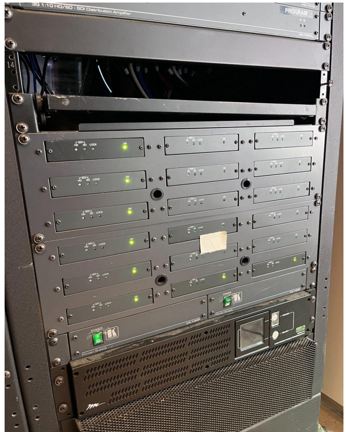
Kramer VM-10HDXL 3G 1:10 HD/SD-SDI DA above a multi-module SDI chassis and lower utility/power equipment.
