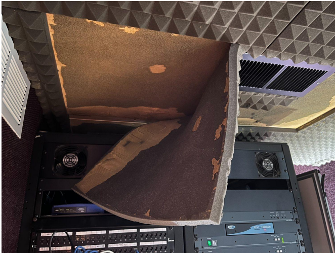
Large acoustic foam panel hanging away from the ceiling/wall substrate.
